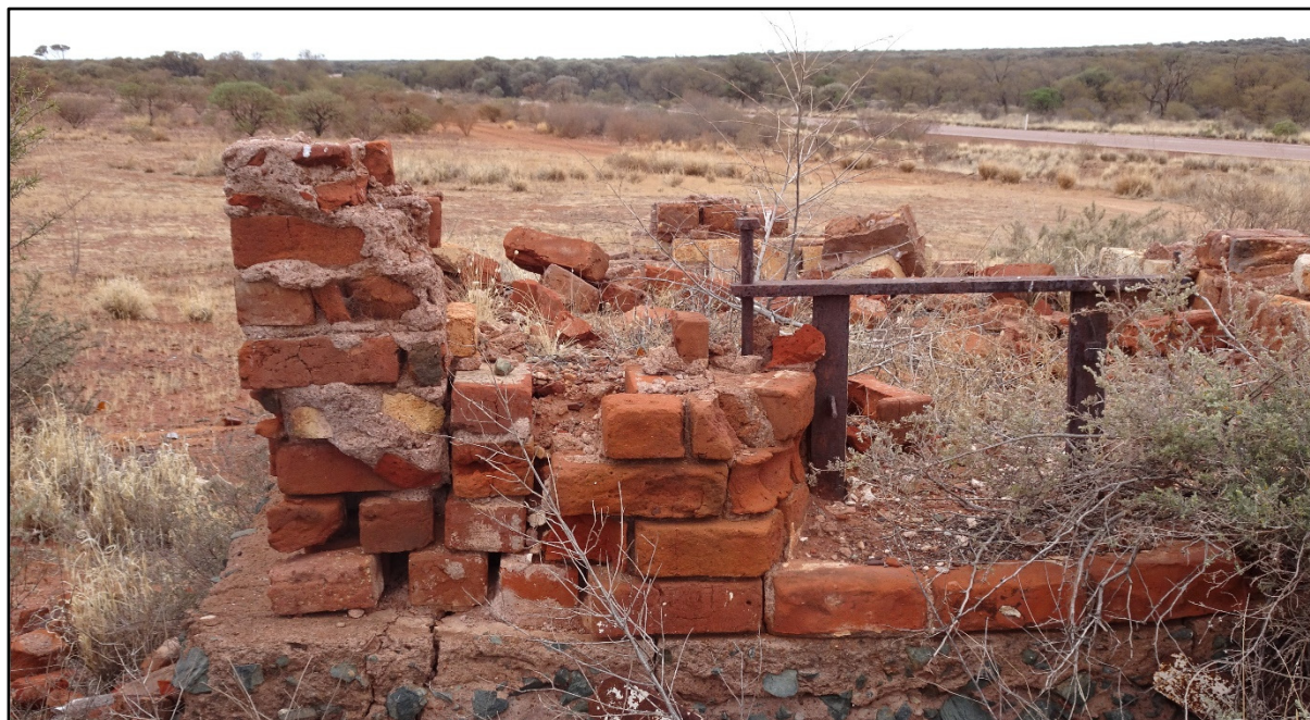
Figure 12: Remains of a brick structure. ID427.
