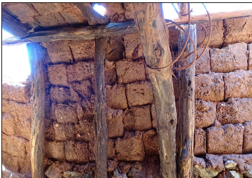
Figure 51: The roof of the hut, made of overlapping, well-made adobe blocks. ID737.
