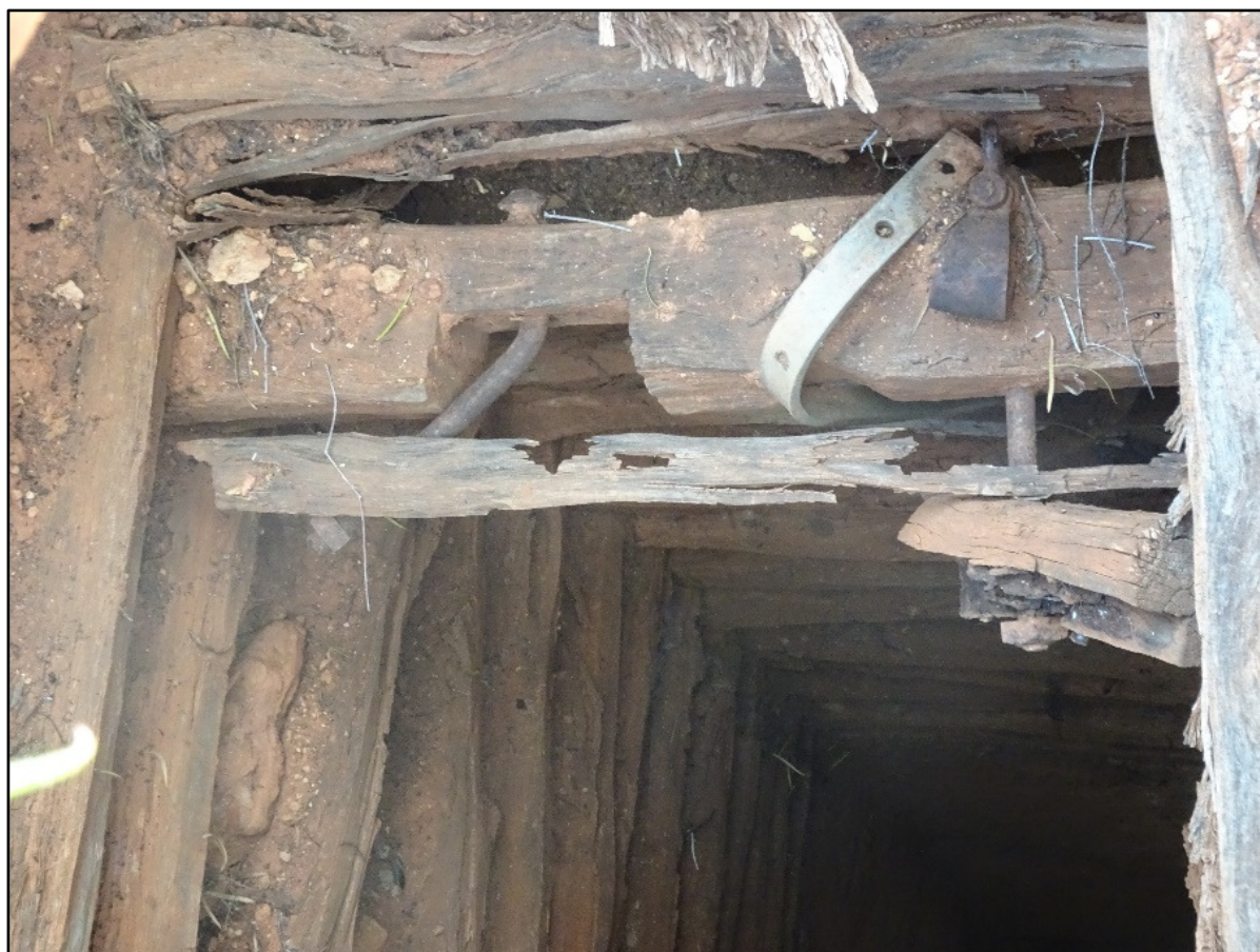
Figure 55: The water well, lined with bush wood, and a bracket most likely for a pump spear. ID455.
